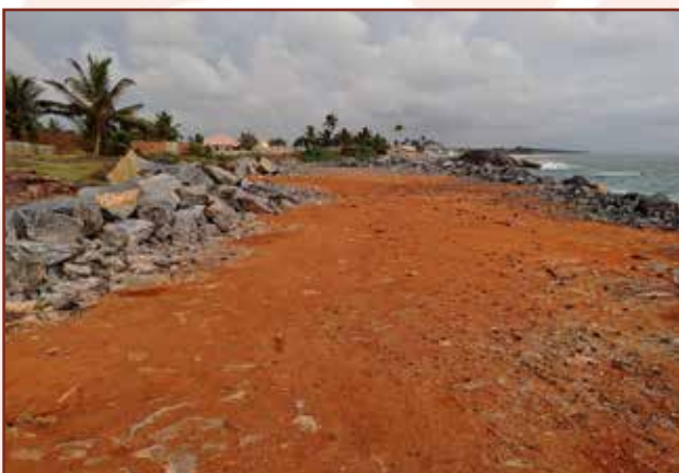
Unnecessary sea defence; beautiful rocks got buried in concrete.
