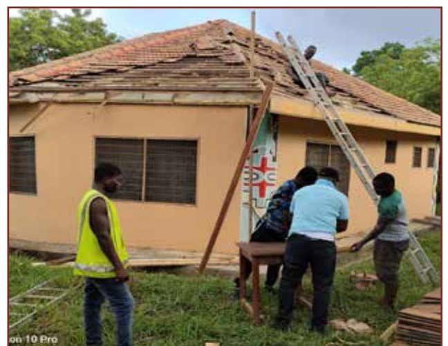
The roof was damaged and in danger to collapse.
